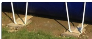
Pavers cracked in half under the load.
