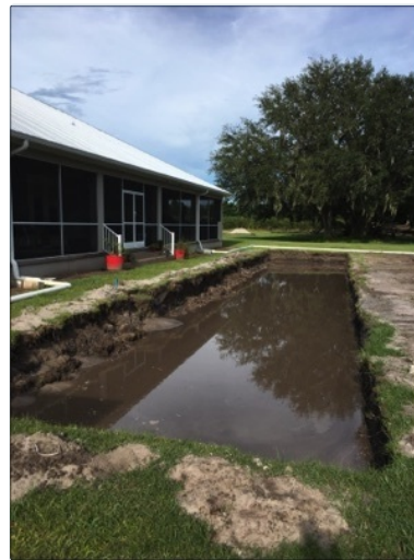
The same hole — groundwater seeping in.
